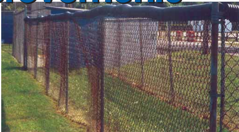
This league fixed the curling bottom edge of this fence before someone was injured.
